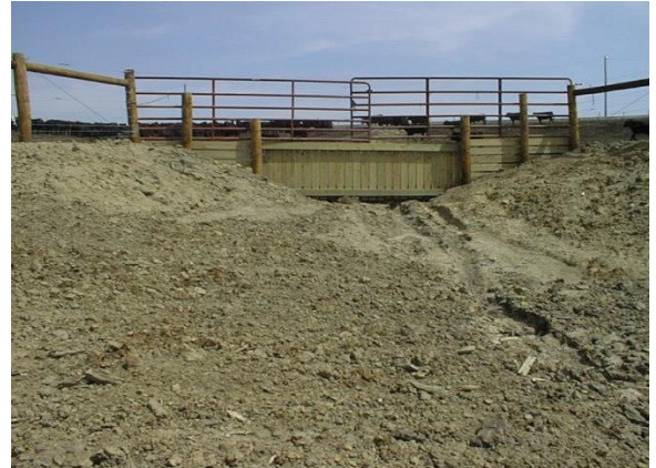
Runoff can cause gullies to form below solids settling structures, especially when the area has been newly seeded. Using mulch or erosion control blankets can reduce channelizing.
